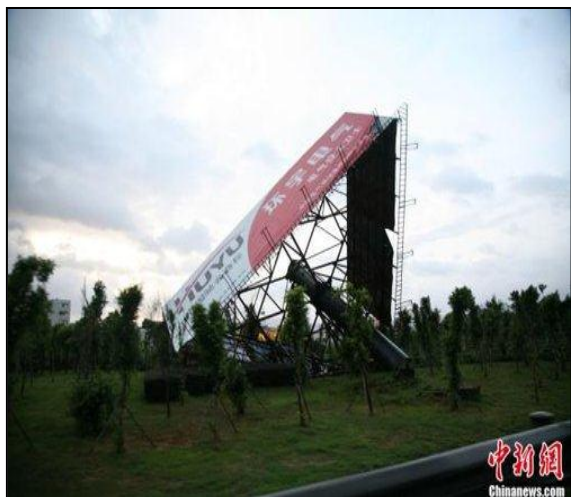
Fig 1.7c: A big billboard damaged by SAOLA
